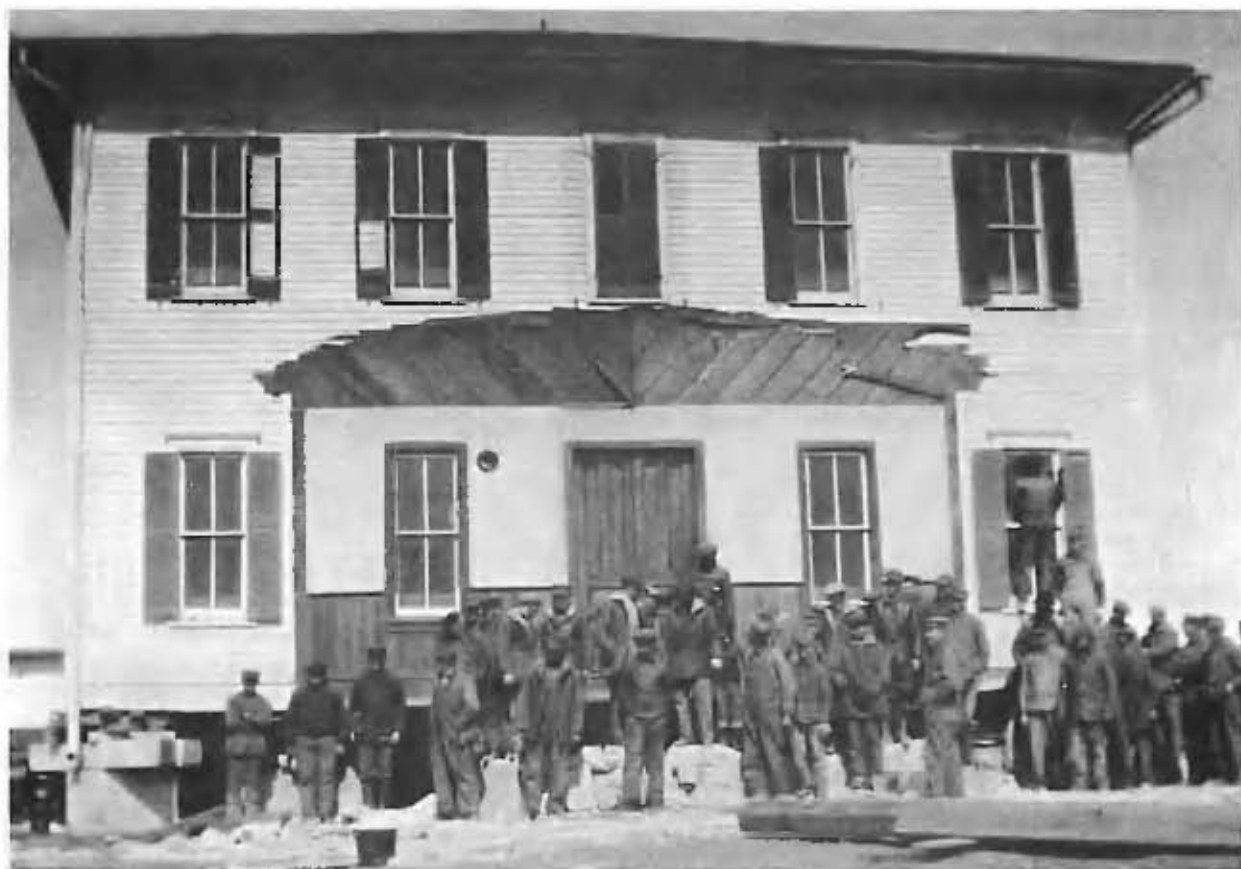
In early 1928, the wings of the Alexanderwohl Church were removed and the structure raised 39 inches in preparation for remodeling.
